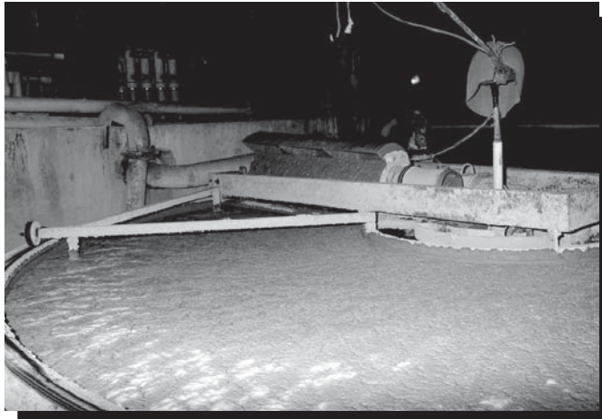
Effluent Treatment Plant
