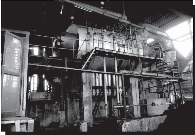
3MW Co-Generation Power Plant - Unit II
