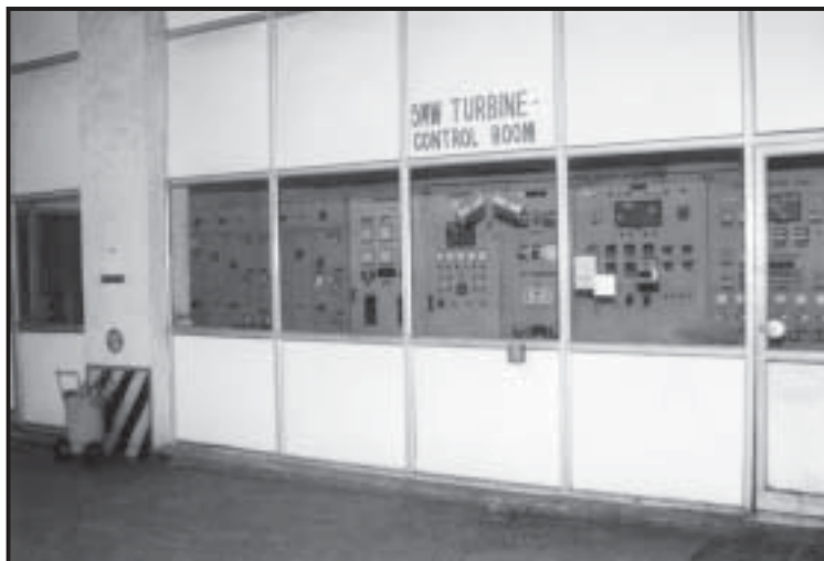
5MW Turbine Control Room
